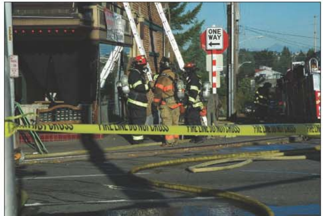
Fig. 10–25. Company officers of the roof ventilation team quickly review assignments before going up the ladder. Understanding the high and low workload positions during a roof operation increases the effectiveness of the team. (Courtesy of Yukari Horikawa)
