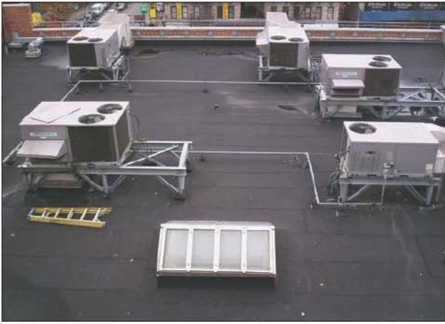
Fig. 14–80. Heavy equipment on the roof—this information should be relayed to the I.C.
