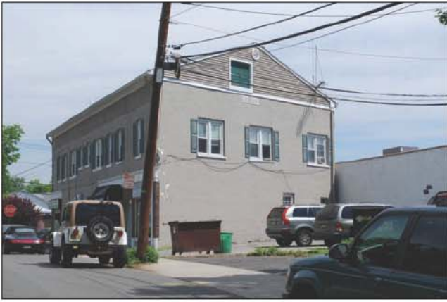
Fig. 14–47. During some building renovations, peaked “rain roofs” are sometimes added over existing flat roofs, which makes ventilation operations difficult.
