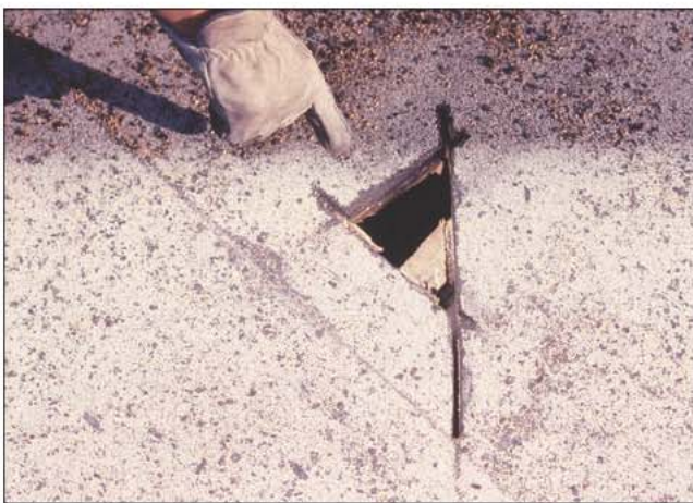
Fig. 14–57. An inspection hole can be used to indicate the type of roof, size of structural members, thickness of the roofing material, and the presence of any fire or smoke. Limit the size of the inspection hole to avoid stepping in it.
