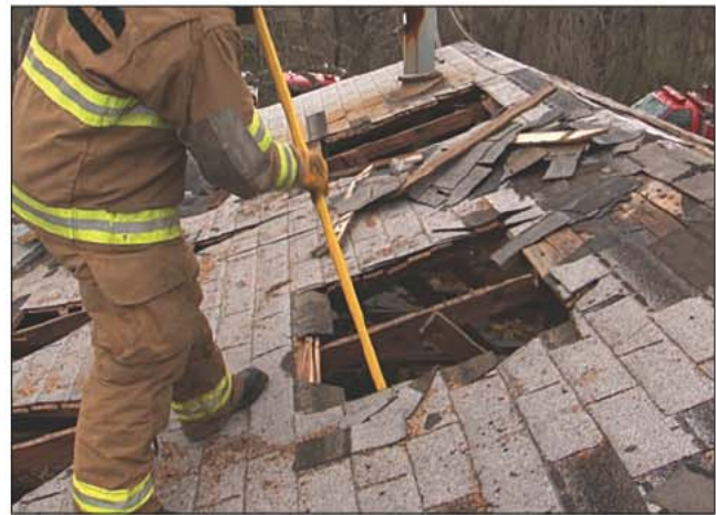
Fig. 14–51. After cutting the roof and removing the sheathing, the task is completed when the ceiling is pushed down.
