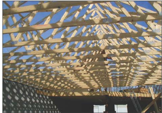
Fig. 14–65. Lightweight wood truss roofs make up most of the new construction today. (Courtesy of Emergency Training Solutions)
