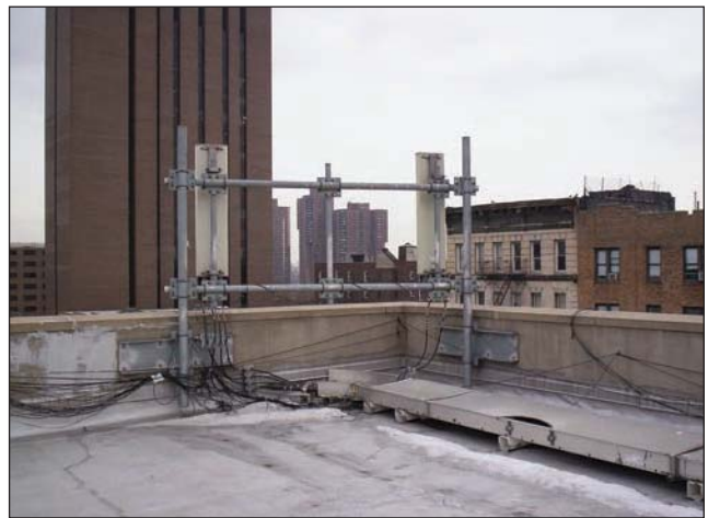
Fig. 14–46. Cell site antennae add more risk from RF wave radiation, which can be dangerous or fatal if standing within 10 ft while transmitting. Look for cell site installations on tall buildings or buildings built on high ground in your district.
