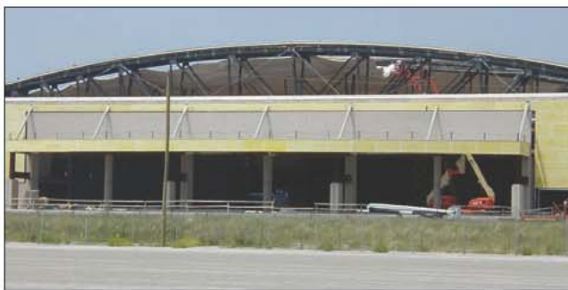
Fig. 14–67. Bowstring truss roofs can be dangerous for firefighting operations. (Courtesy of ETS)
