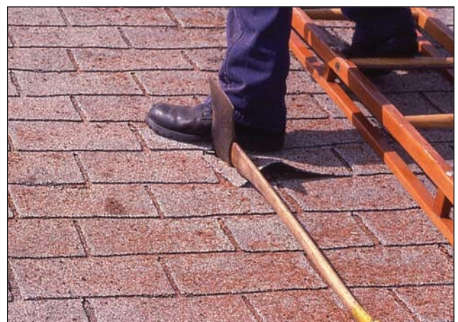
Fig. 14–53. A tool such as a pick-head axe can be driven into the roof as a safety step while working on a peaked roof.
