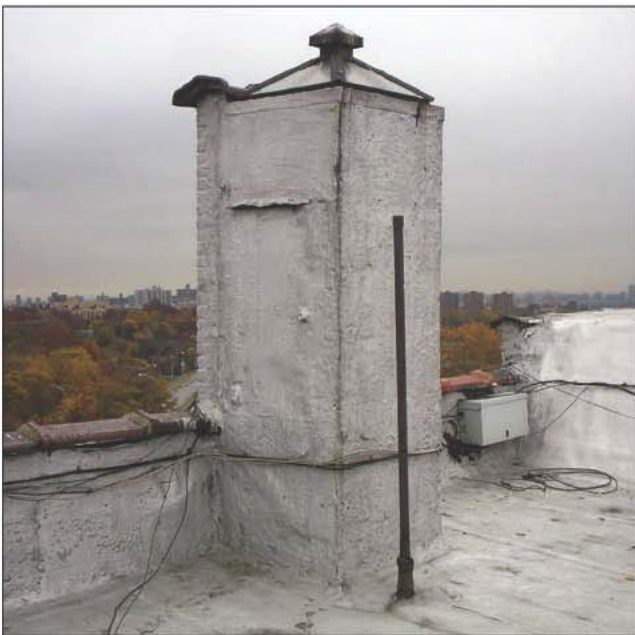
Fig. 14–26. There are many avenues for fire to travel horizontally, as well as places to perform ventilation, such as this dumbwaiter bulkhead.
