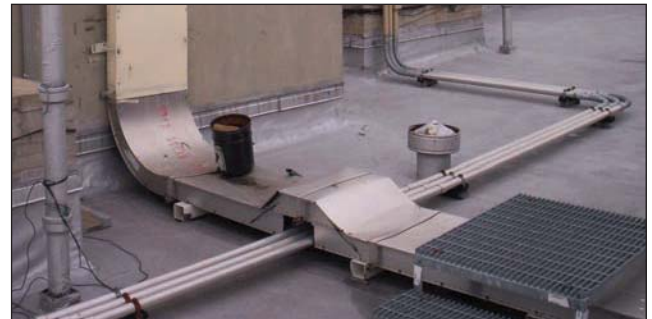
Fig. 14–4. Caution should always be used when working around electrical lines. They are just one of many hazards on rooftops that can have fatal consequences.
