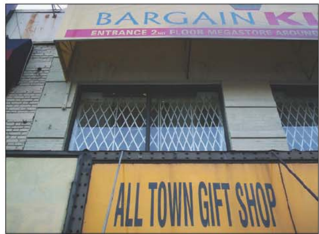
Fig. 14–39. Although typical in residential multiple dwellings, scissor gates can be found in commercial occupancies as well, and will delay egress through these windows.
