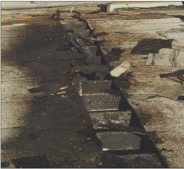
Fig. 14–61. A trench cut must extend from one side of the building to the other side and be wide enough to stop the spread of fire.
