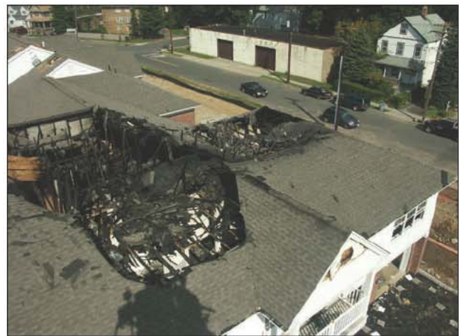
Fig. 14–66. There is considerable danger involved in working on or under roofs with severe fire.
