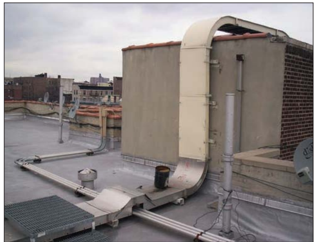
Fig. 14–45. Cell site equipment introduces new hazards to roof operations.
