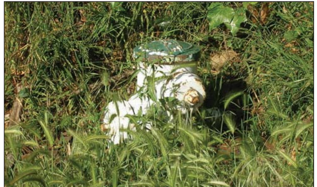
Fig. 15–14. This hydrant needs to be dug out and have the vegetation trimmed to ensure access when needed.
