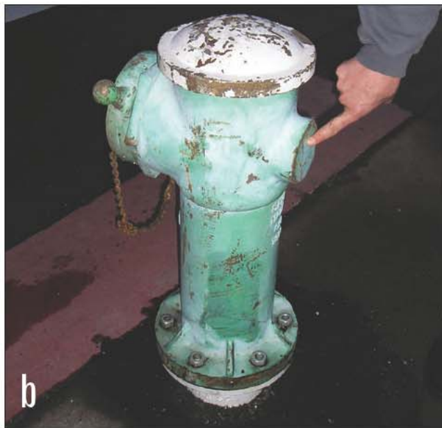
Fig. 15–19 a, b. A drafting hydrant allows the fire service to easily access an untreated water source. Notice that there is no operating spindle on the hydrant.
