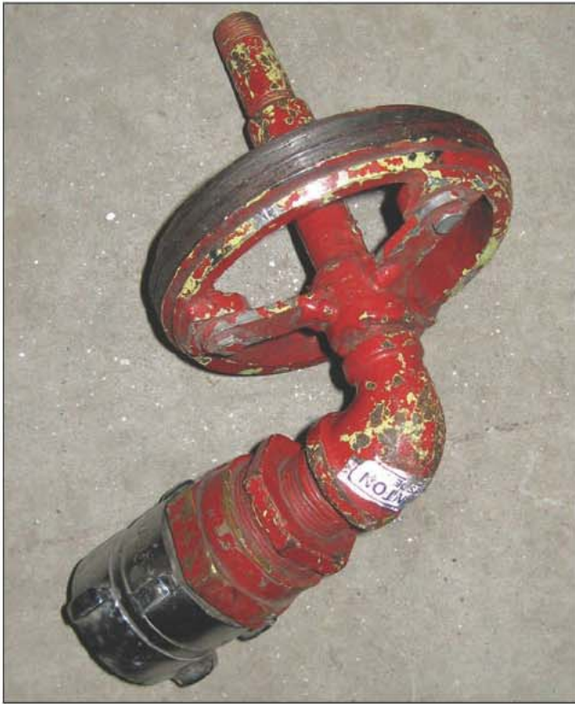
Fig. 15–20. Jet siphons are typically used to move water from one portable tank to another.
