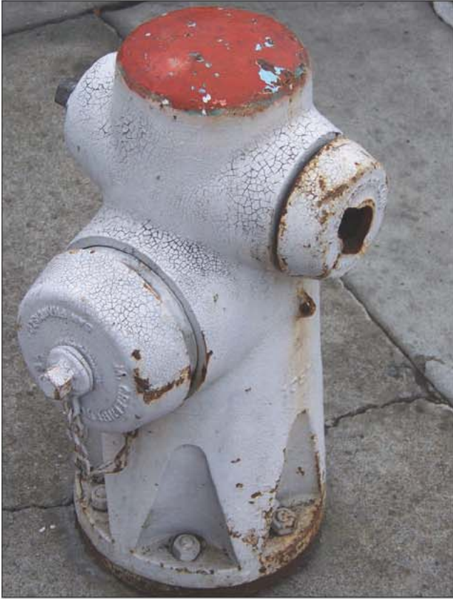
Fig. 15–15. This hydrant is missing a cap nut and chain.
