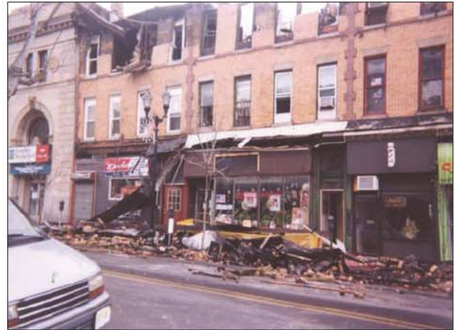
Fig. 17–12. This collapse occurred several hours after fire operations ended. Fire watch was still on scene. The risk was evaluated, and control measures were taken by cordoning off the area, which kept personnel away from the danger. No one was injured.
