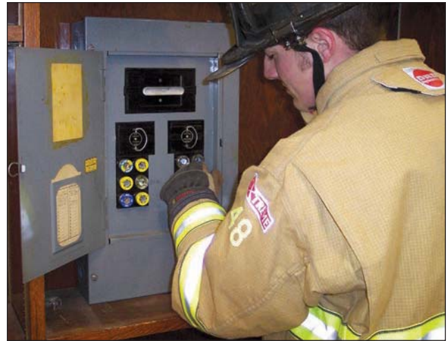
Fig. 17–38. A fuse box
