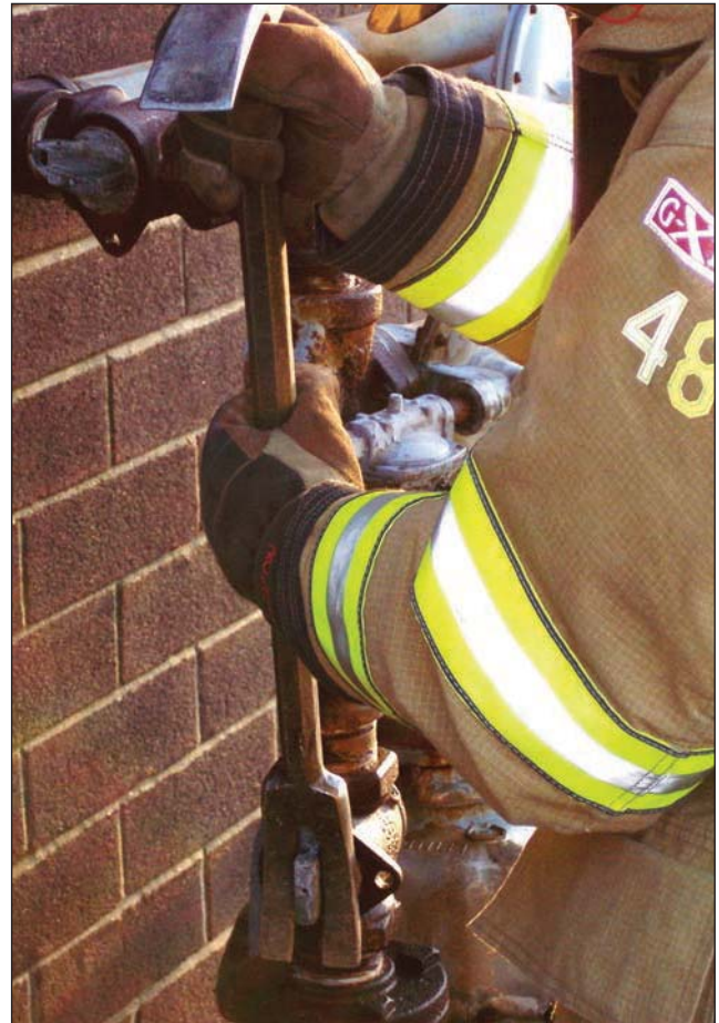
Fig. 17–39. A gas meter with a gas cock
