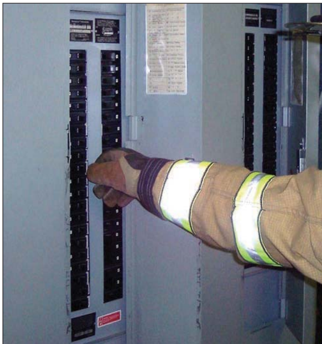
Fig. 17–37. An electrical panel with circuit breakers
