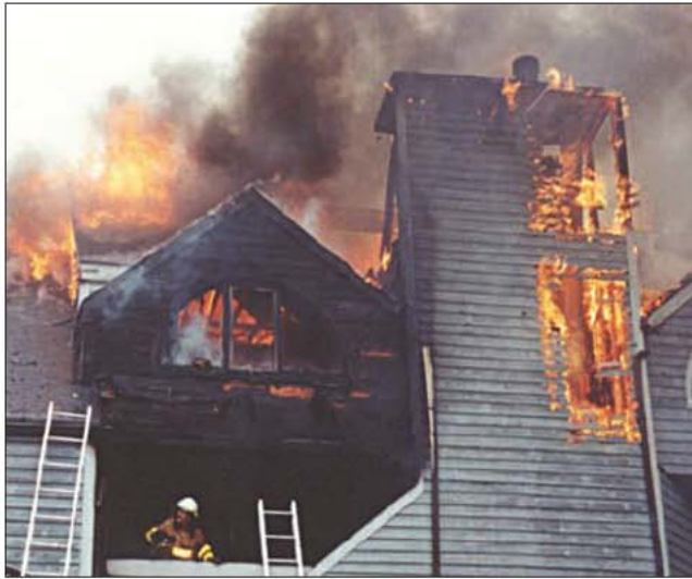
Fig. 17–53. The truss above this firefighter's head is clearly involved in fire. This is a tragedy waiting to happen. (Courtesy of BC Mike Oriente NHRFR)
