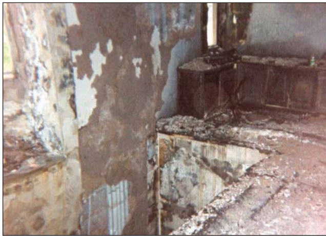
Fig. 17–50. Photo of the shaft that author Frank Ricci fell into when searching for a trapped security guard. Make sure that if you encounter a shaft, you can pull yourself back up.
