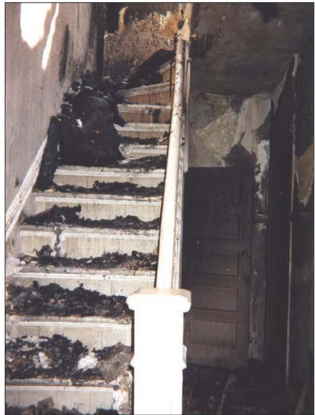
Fig. 17–60. Fire roaring up the stairs from the cellar trapped firefighters searching above the fire. Only a closed apartment door protected them from burning to death. In private dwellings, this apartment door is not available.
