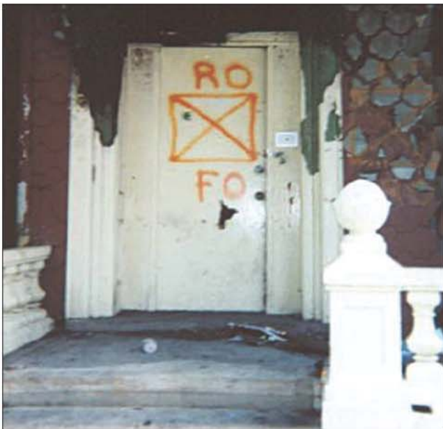
Fig. 17-74. Hazardous vacant building (HVB) markings on this building prohibit entry as well as bring attention to hazards created by an open roof and floor. This is a Level 3 hazardous vacant building. Marking systems such as this allow a fire department to alert its firefighters to the dangers before they enter a building.
