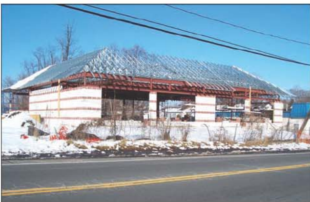
Fig. 20–71. Note the lightweight and unprotected C channel members holding up the roof.
