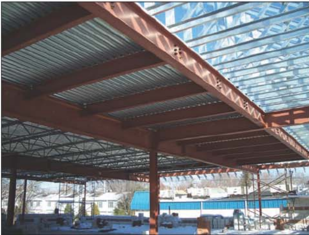
Fig. 20–70. Unprotected steel structural members will fail rapidly under a fire load.
