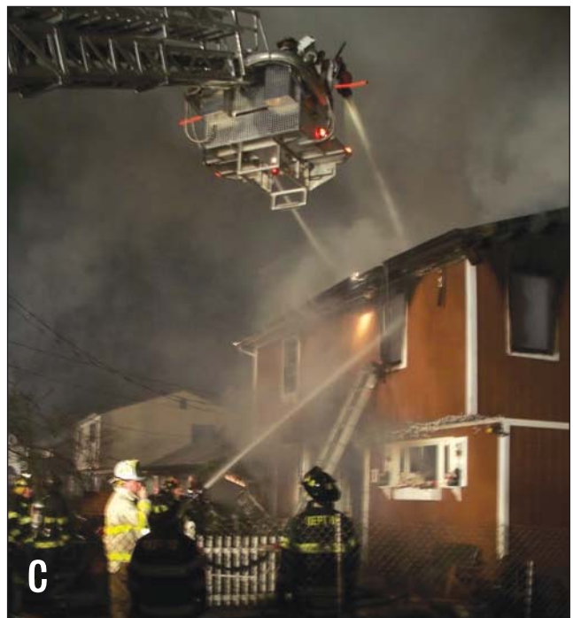
Fig. 20–10. a) This fire started out as an offensive attack. b) Heavy fire conditions inside combined with a large amount of accumulated materials inside the house prevented the interior attack lines from advancing and thus forced firefighters to change from an offensive operation to a defensive attack. c) The fire was contained with no injuries to firefighters.
