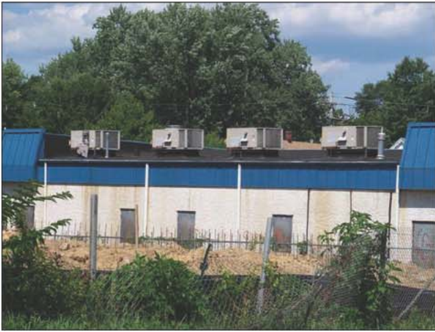
Fig. 20–69. The rear of the building provides limited access and usually high security. Note the roof-mounted HVAC units. (Courtesy of J. Knapp)
