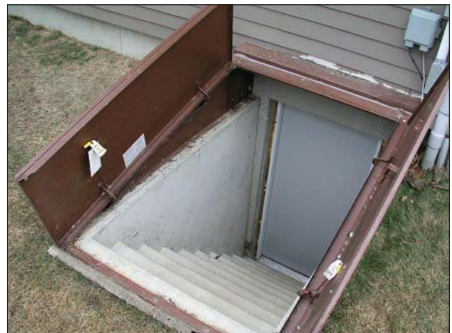
Fig. 20–64. Clamshell doors provide exterior access to basement.
