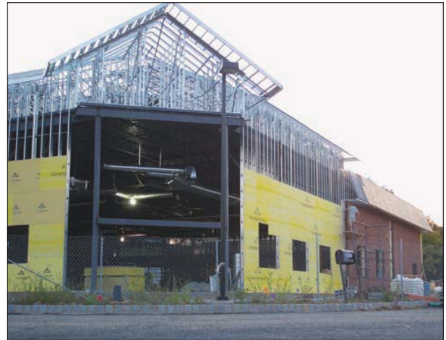
Fig. 20–72. Note the lightweight construction, unprotected steel, and large size of this building.
