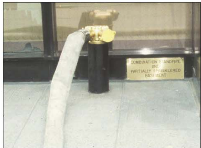
Fig. 20-46. Hoseline attached to a standpipe Siamese connection
