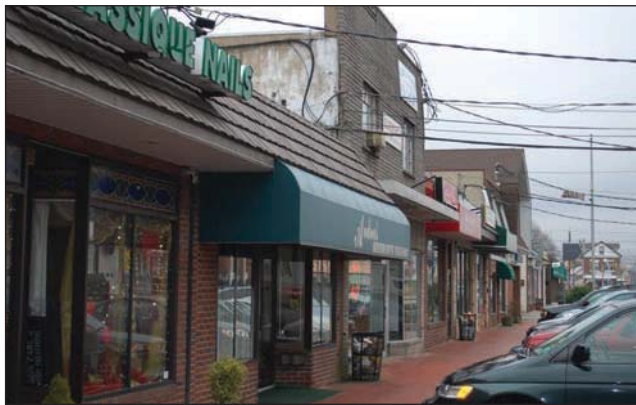
Fig. 20–66. This taxpayer's parapet is leaning and may be unstable.
