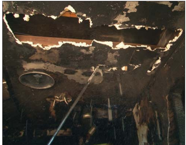
Fig. 21–19. The ceiling punch technique involves using a pike pole to weaken gypsum board so that it can be removed more easily in large pieces.
