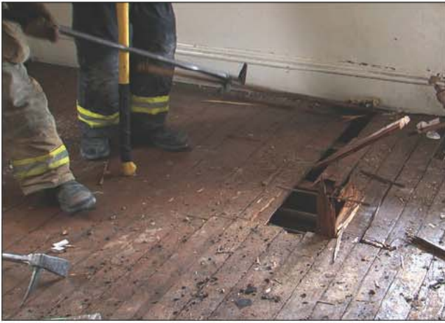
Fig. 21–22. When opening up floor assemblies, firefighters must be careful not to cut through the beam below, compromising its load-carrying capability.
