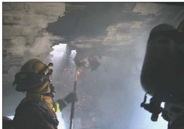
Fig. 21–17. Numerous toxic gases are produced during the decay stage of a fire, when overhaul takes place. Therefore it is imperative that firefighters always wear SCBA.
