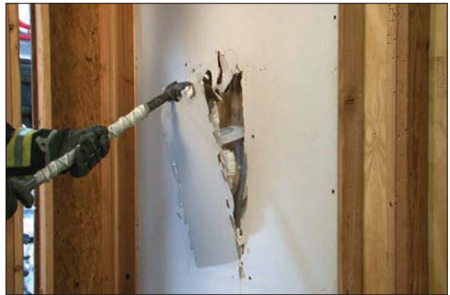
Fig. 21–20. The wall punch technique works in a similar manner to the ceiling technique. However, the tool of choice for this evolution is the Halligan.
