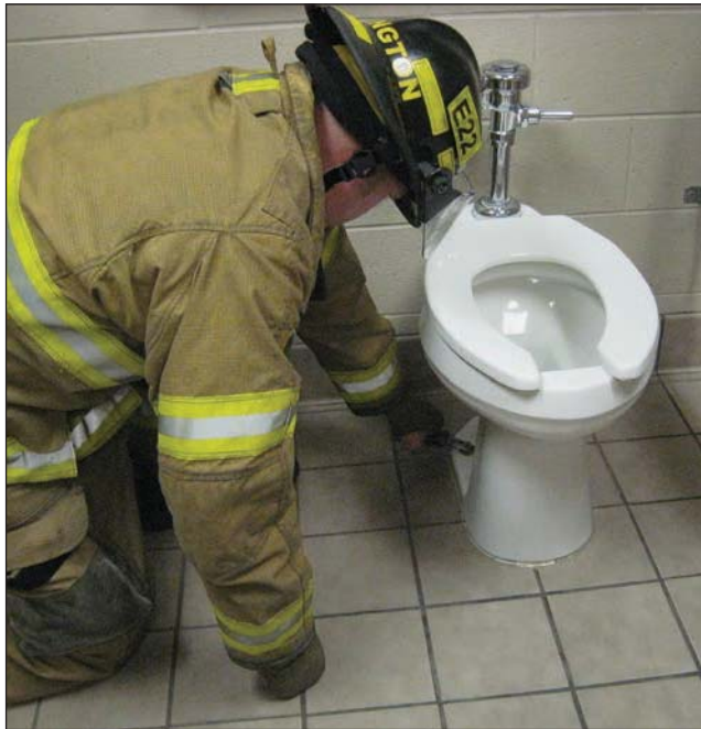
Fig. 21–9. To facilitate draining, a toilet can be removed. This tactic can be especially important in multi-story buildings where creating chutes and catchalls isn't feasible.
