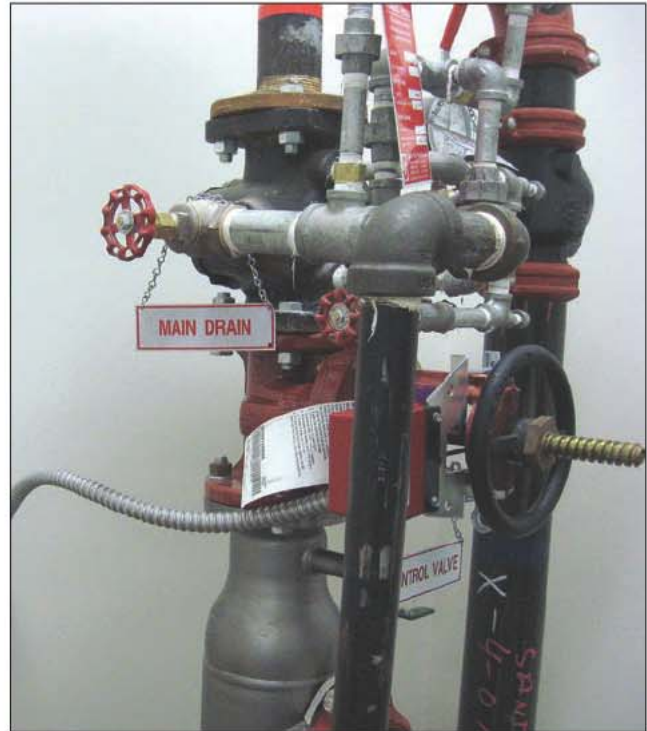
Fig. 21–14. The main drain of a sprinkler system is normally labeled and easy to locate.
