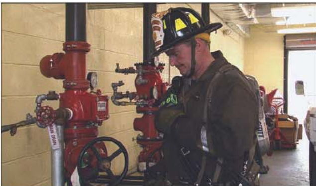
Fig. 21–13. An outside stem and yoke (OS&Y valve) in the “closed” position
