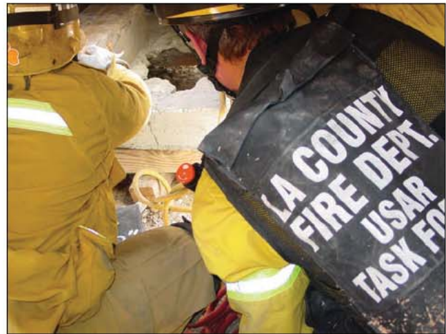
Fig. 35–35. Firefighters must be prepared to assist technical rescuers with gathering equipment and shoring materials for complex structural collapse incidents.
