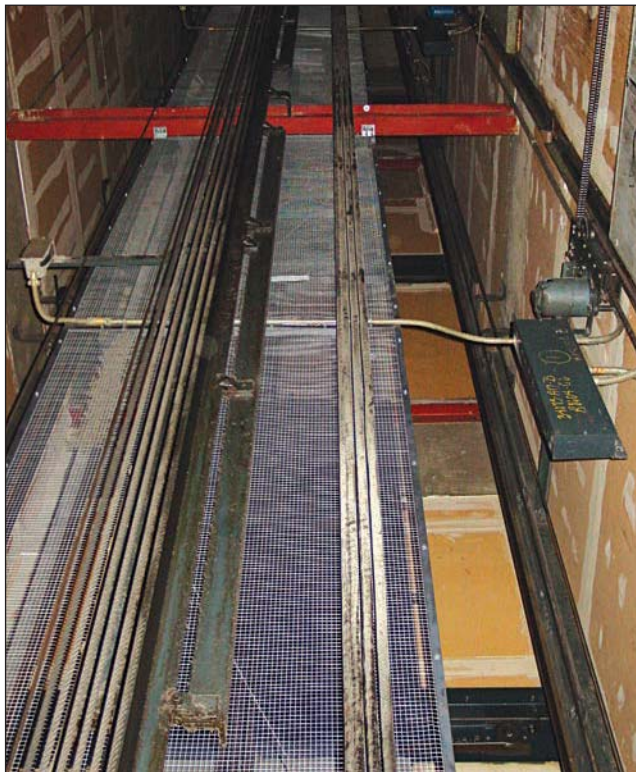
Fig. 35-83. Firefighters can determine the location of an elevator through the top or bottom of the elevator shaft.
