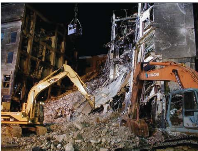
Fig. 35–39. Removing debris from a collapsed structure to a safe area is a difficult task, but one common for the firefighter.
