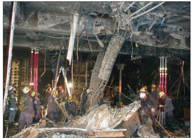
Fig. 35–38. Once supplemental shoring is placed in a building, it should not be removed, as it may cause secondary collapse.
