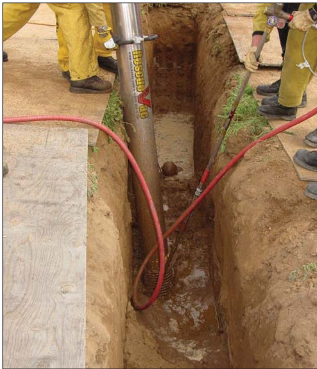
Fig. 35–61. Controlling utilities, especially water service, is of extreme importance during trench operations.
