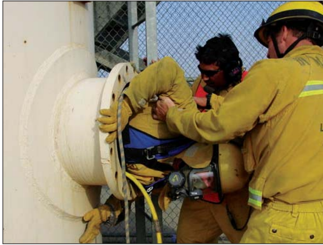
Fig. 35–65. Restrictive ingress and egress openings in confined spaces present a large risk to rescuers.
