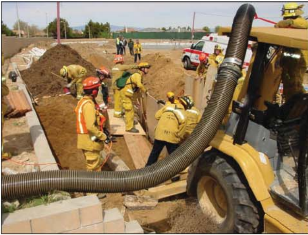
Fig. 35-58. Edge protection along the sides of the trench can help distribute weight and prevent secondary collapse.
