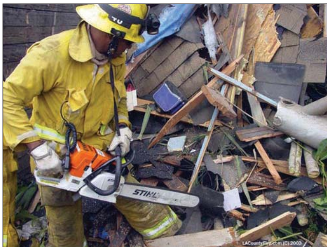
Fig. 35–27. A chainsaw can assist rescuers in gaining access to victims trapped beneath collapse structures.
