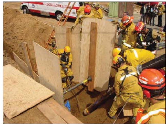
Fig. 35–56. Trench and excavation emergencies involve rescuing victims from below grade earth cave-ins.
