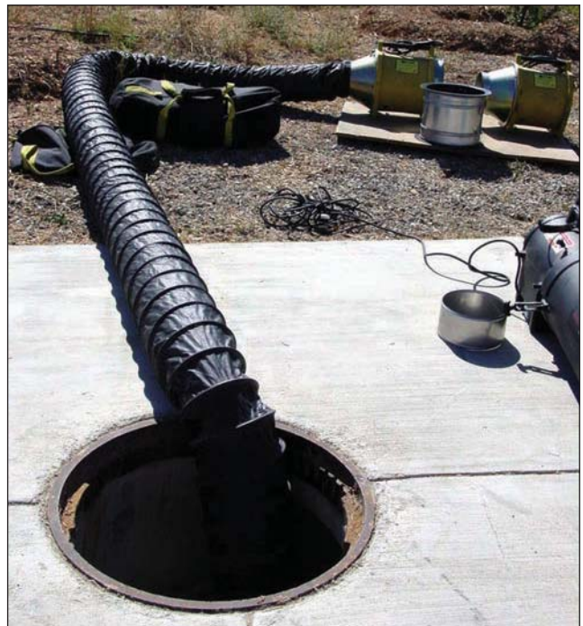
Fig. 35–72. Ventilation of the confined space can help alleviate a hazardous atmosphere and can make the space more tenable for the victim.
