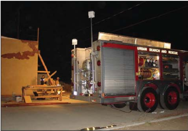
Fig. 35–22. Technical rescue apparatus should be placed as close to the collapsed structure as can safely be arranged to aid in tool accessibility.
