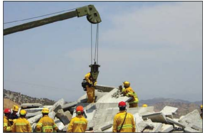
Fig. 35–40. Dismantling the collapse zone through selective debris removal is part of stage 4 operations.
