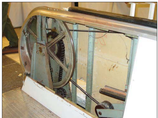
Figs. 35–92 a & b. Cutting through and manipulating belts, as well as moving stairs and other mechanisms can be done to free the victim.
