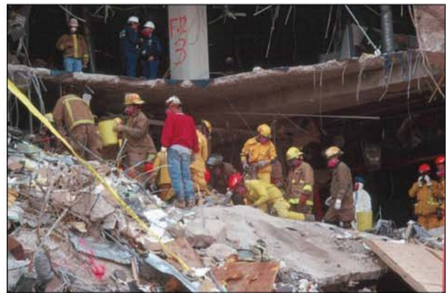
Fig. 35–36. Although it is preferred to have highly trained technical rescuers conduct structural collapse searches, under extraordinary circumstances firefighters may have to undertake these responsibilities.
