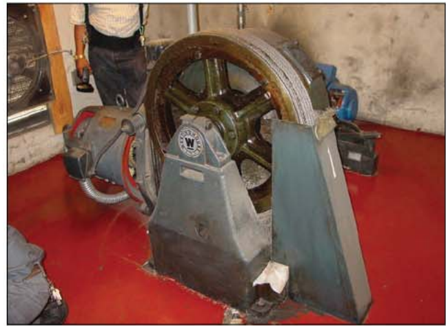
Fig. 35–82. Motors for elevators are typically located in a designated elevator machinery room inside the building.
