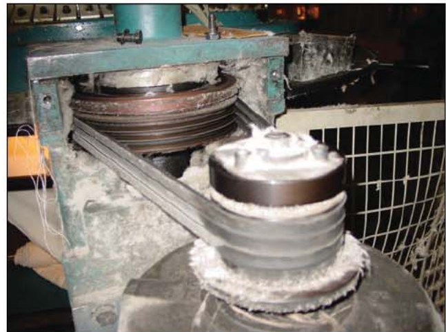
Fig. 35–79. Stabilizing and securing belts, pulleys, and other moving parts are essential since some machines may have trapped a victim during the middle of a cycle, thus presenting a further hazard as the person is freed.
