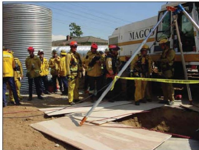
Fig. 35–73. Plywood or other decking material should be placed around the edges of the entrance.
