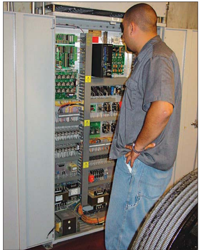
Fig. 35-84. Securing the electrical service to the elevator can be done by a trained firefighter or by a building maintenance person.
