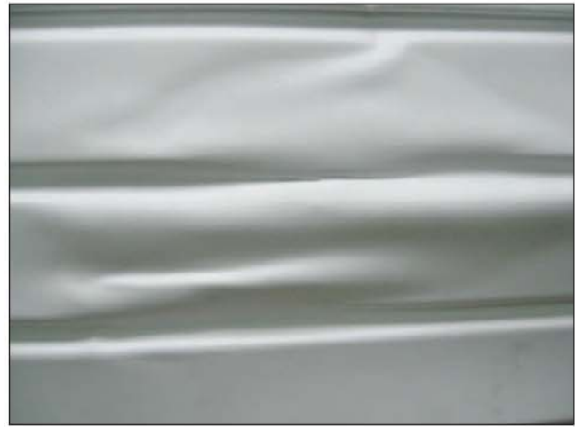
Fig. 5–9. Vinyl siding melted by radiant heat
