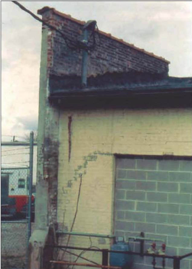
Fig. 7-16. Freestanding parapet walls are the most dangerous parapet walls, as they do not intersect at any corner. If the roof of the building were to collapse during a fire, the freestanding portion of the wall may become greater and therefore less stable.
