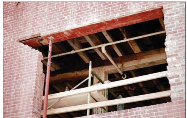
Fig. 7–31. In this photo, a mill building is being renovated and a window is being added in the exterior wall. Notice the thickness of the exterior wall, the size of the interior column, beam, and floor joists. The original building had no ceiling other than the underside of the floor above. If during the renovation a ceiling is added under the floor joists (this is not permissible under most building codes), a combustible void space will be created. (Courtesy of William P. Dansbach)
