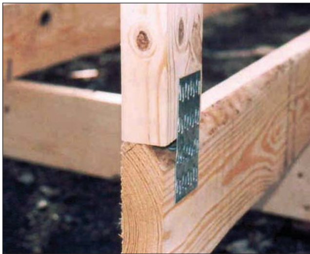
Fig. 7-44. The lack of quality control has led to the truss being delivered to the construction site with one entire row of the connecting teeth of the gusset plate not being secured into any part of the wood truss. The heat from a fire will quickly attack these connections; this connection being less secure than the remaining gusset plates is likely to fail very early in the fire.
