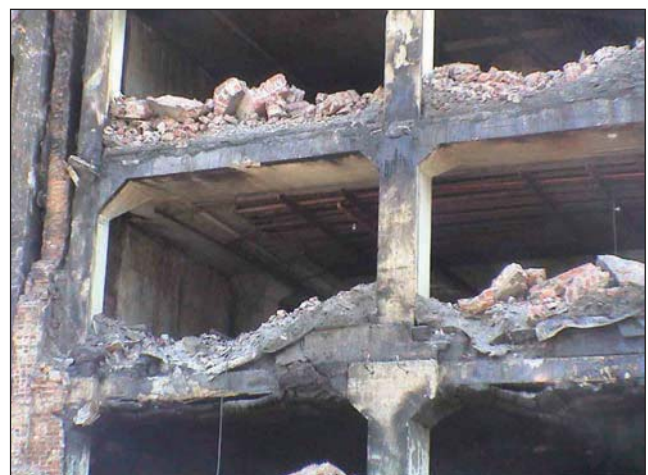
Fig. 7–20. A poured-in-place fire-resistive constructed building. This construction is also sometime called monolithic construction as the poured concrete forms into one piece. Detailed here are the building columns and floor assemblies, poured into the concrete columns and floor steel reinforcing bars. (Courtesy of Glenn Taldelore)
