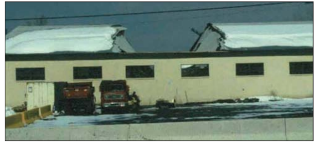
Fig. 7–10. An unusually heavy snow load caused the collapse of this bowstring truss roof. The fire department was dispatched to this collapse as an activated fire alarm. When the collapse occurred, the building's automatic sprinkler piping was broken and the resulting water flow tripped the fire alarm system. Note the large area of collapse as the result of the failure of only one of the bowstring trusses.
