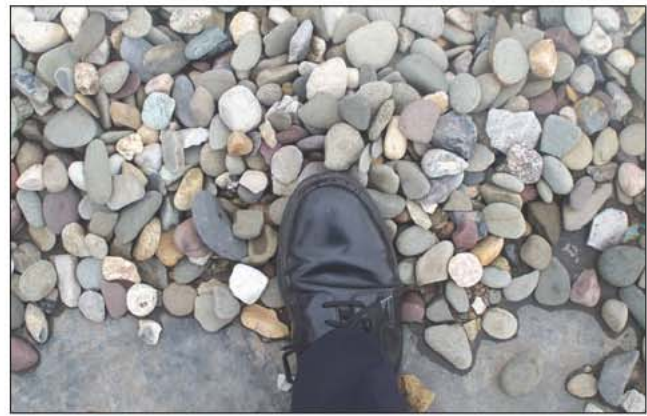
Fig. 7–45. The ballast stones are placed on the roof to prevent the roof covering from lifting and are not secured to the roof. These stones make footing on these roofs difficult. The stones also add weight to the roof structure and create surface tension that slows down the drainage capability of the roof.
