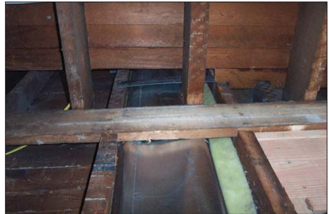
Fig. 7–35. In a building that is balloon framed, the exterior wall studs run from the basement to the attic without fire stopping. This photo looks up the wall as it passes the second floor joists; note the lack of fire stopping and the ease with which the duct work was run in the wall. This vertical void space becomes a chimney for the fire to travel from the basement to the attic.
