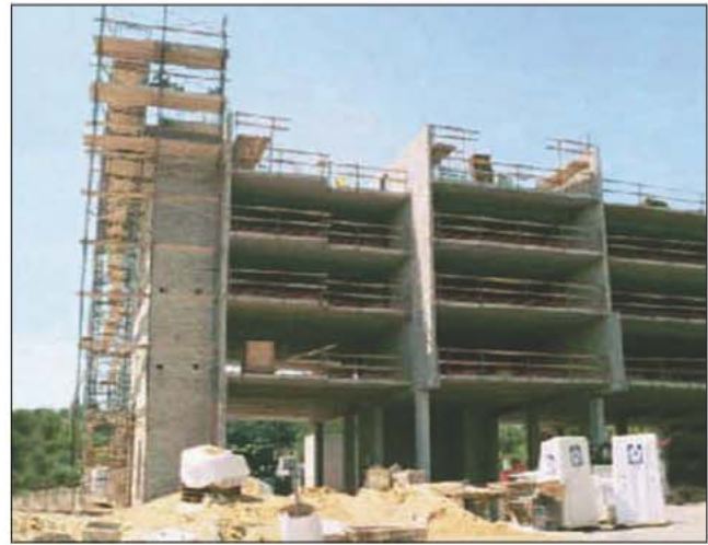
Fig. 7–22. Fire-resistive constructed hotels will have the greatest amount of compartmentation because the size of the hotel room will limit the fire area. In this photo the space between the block walls will be further reduced by a non-bearing wall sub-dividing the space into two hotel rooms between the block walls.
