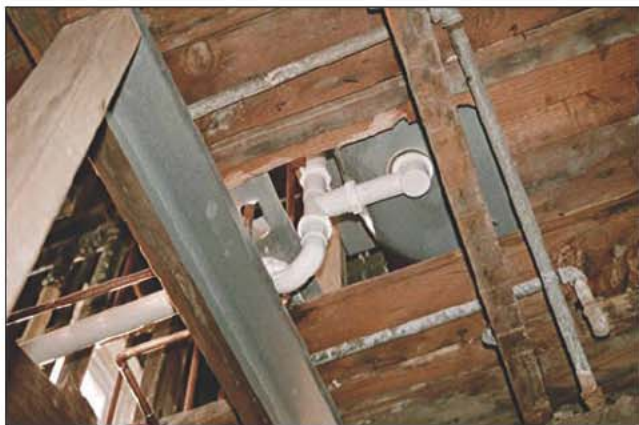
Fig. 7–28. There is no fire-stopping or blocking installed around the bathtub waste line on the floor above. From the floor below, we can see the bottom of the bathtub. Fire that starts or extends to the combustible ceiling/floor space will rapidly extend vertically through the building.
