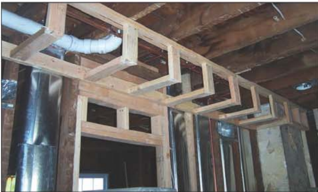
Fig. 7–41. A kitchen renovation that results in the creation of combustible void spaces when the framing for the cabinet soffit has been installed without first installing drywall on the wall and ceiling behind the soffit. Should the fire extend into the combustible void space created by the soffit, the fire will extend horizontally throughout the soffit and vertically in any non-fire-stopped void spaces in the wood framing.
