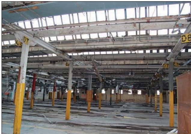
Fig. 7–29. A typical floor of a mill or heavy timber building; notice the large cross-section dimensions of the columns and beams, the wide-open area that permitted the movement of goods and materials. This area was also the top floor of the building as evidenced by the rows of skylights that allowed natural light to enter the building. (Courtesy of William P. Dansbach)
