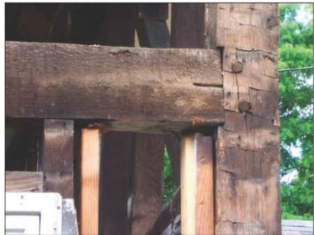
Fig. 7-33. This photo details the mortise and tenon connection where the post is connected to the beam, the connection is secured with dowel-like pegs called trunnels . The mortise and tenon connection is the weakest point in the framing system as 2/3 of the mass is removed from the beam and 1/3 of the mass is removed from the post to create the connection. (Courtesy of Tim Hetzel)
