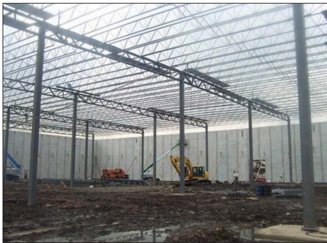
Fig. 7–23. A one story, non-combustible warehouse under construction. The roof system is supported by unprotected steel columns and bar joist trusses. These buildings are very prone to early collapse as the heat of the fire attacks the steel and the steel reaches its yield point and fails.
