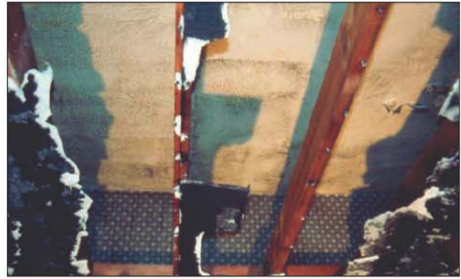
Fig. 7–42. A dropped ceiling of 2 x 4s and drywall has been constructed below the original plaster and lathe ceiling. When checking for fire extension, firefighters must recognize this feature and continue to open the ceilings until they have exposed the underside of the floor or roof above. In this photo, the task was not completed as only the dropped ceiling has been removed leaving the plaster and lathe ceiling intact.
