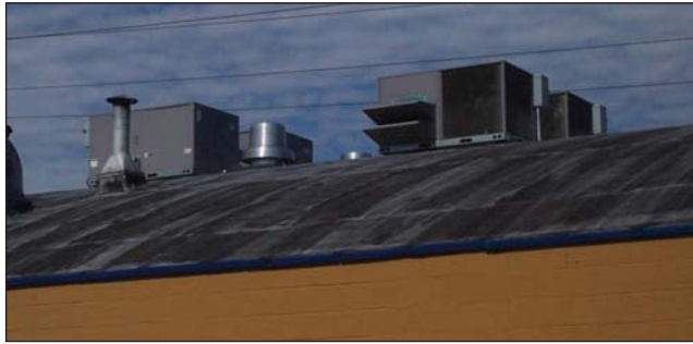
Fig. 7–9. The installation of air conditioning units on a roof without consideration of the extra weight being added to the roof is an example of an undesigned load.
