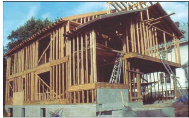
Fig. 7-37. In a building constructed of platform-frame construction, each story is built on top of the floor below. Notice the floor joists of the first and second floors extend to the outer edge of the framing, creating inherent fire stopping. (Courtesy of Robert Moran)
