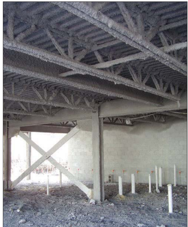
Fig. 7–19. This photo details the use of a spray on fireproofing material on structural steel columns and bar joists. The material is a mixture of an insulating material and cement. The cement binds the insulation together and ensures that the fireproofing adheres to the building component. This material is easily removed by other construction trades and results in a lapse of protection.
