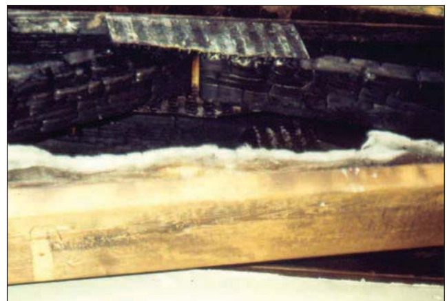
Fig. 7–40. The lack of penetration of the teeth on the gusset plate allows it to warp and twist out of the truss. Loss of strength in the connection will lead to the failure of the truss.
