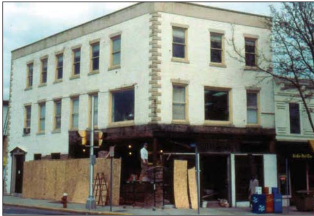
Fig. 7–26. Ordinary-constructed buildings are made of masonry exterior walls, wood joist floors, and a wood roof structure. When the building has a storefront, the opening for the storefront windows is created with columns and beams. The steel columns and beams may be steel or cast iron. In the photo, the columns and beams support the total weight of the second and third floors, the roof structure, and the weight of the exterior masonry walls. (Courtesy of Christian P. Dansbach)
