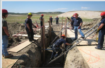
Trench & Excavation Collapse Rescue
