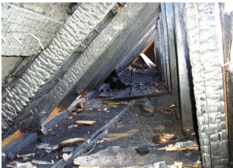
Figure 37. Facade without Fire Stops, notice the uninhibited fire travel.
