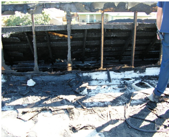
Figure 38. If Facade is involved with fire, ensure that the entire facade is opened up to check for fire extension and stop fire travel.
