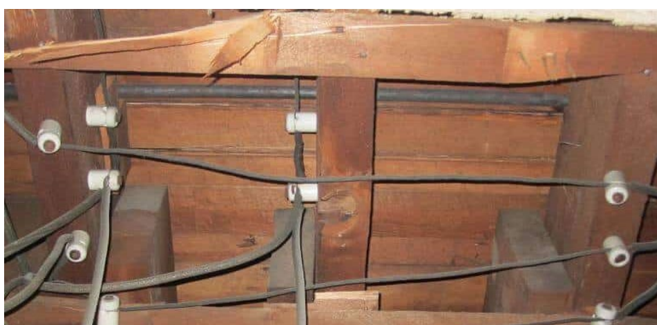
Figure 42. Knob and Tube Wiring
