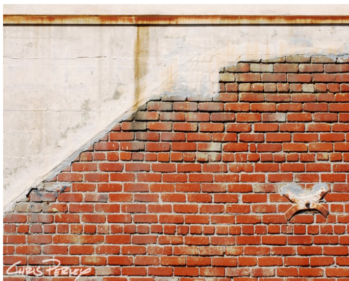
Figure 30. Rafter Tie Plate in Pre-1933 Masonry Brick Construction. Also shown King Rows.
