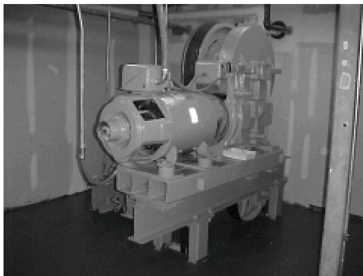
Figure 2 - Traction Elevator Machine Room
