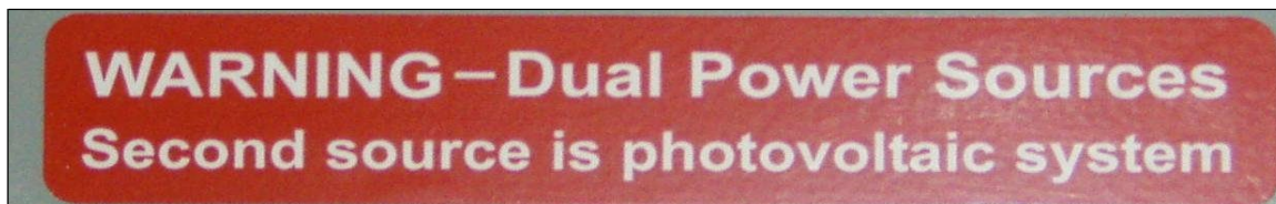
Figure 29 - Warning label on the front of a Main Electrical Service Panel (circuit breaker). The label in this instance clearly identifies the secondary power source is solar PV.
