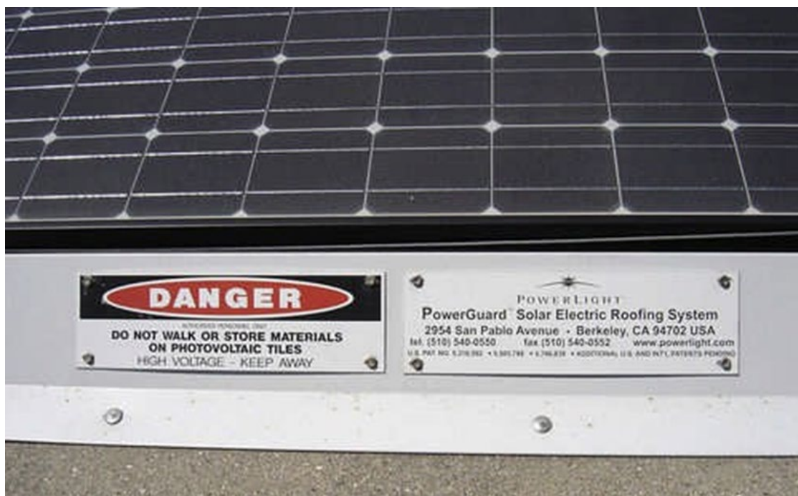
Figure 31 - Label on the side of a solar PV mobile installed on the roof, provides firefighters with a reminder of potential hazards as well as the name of the electrical contractor who installed the system.
