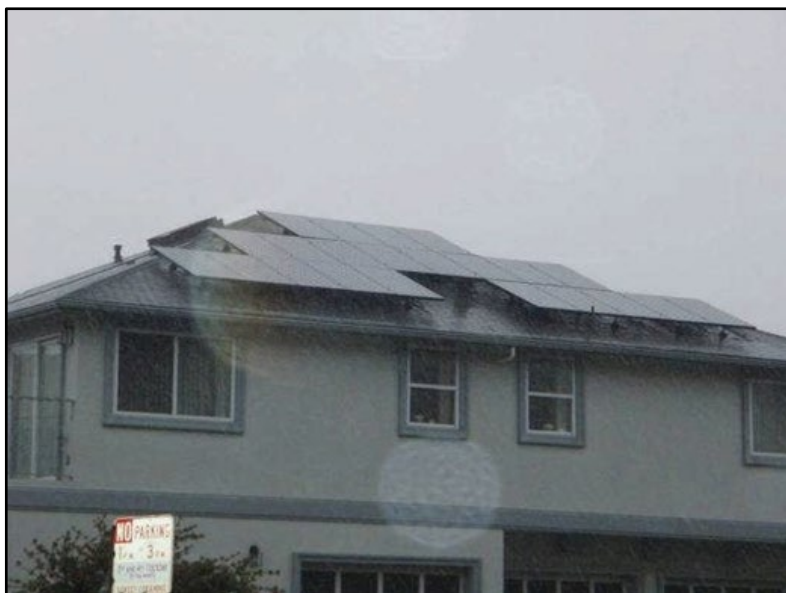
Figure 36 - Roof Top Residential PV System
